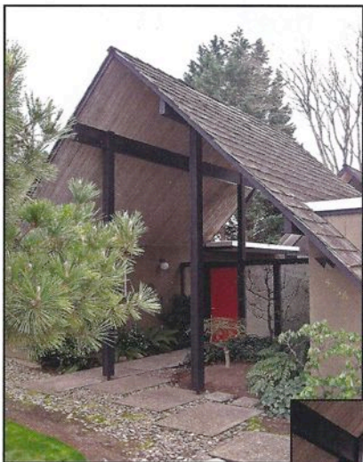
Covered entryway in this Oak Hills Rummer reveals the post-and-beam construction used throughout the house.
